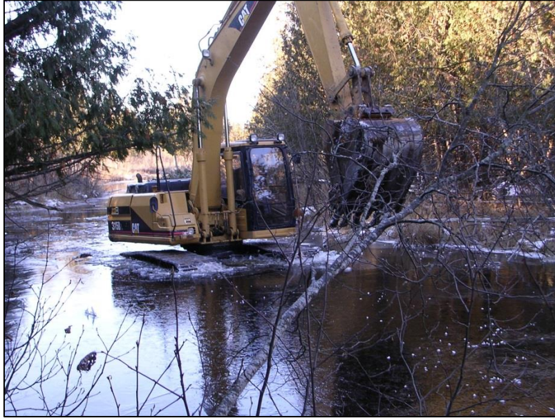
Figure 2. Addition of large woody debris with the use of an excavator occurred in 2003 (Top picture). Placement and position of large woody placed into Hunters Brook (bottom picture).
