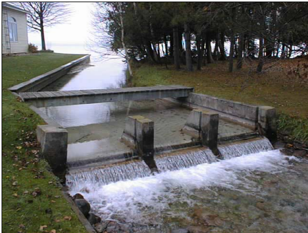
Tressler Dam (North Manistique Lake) at low flow with all boards removed.
