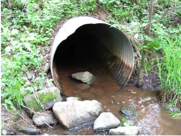
At Stream Grade – bottom of culvert is at or below the elevation of the stream bed.
