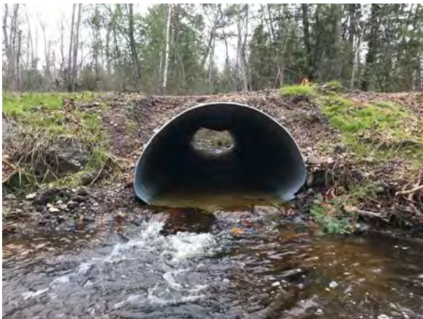
Poor (unprotected embankment slopes)
