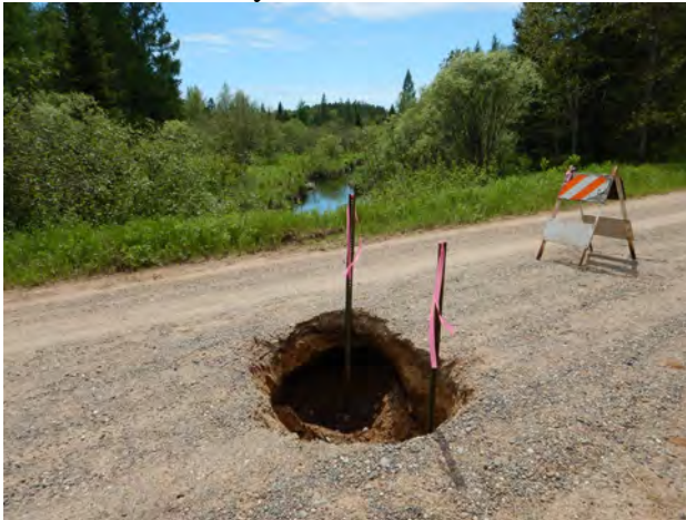
Sink holes directly over the culvert
