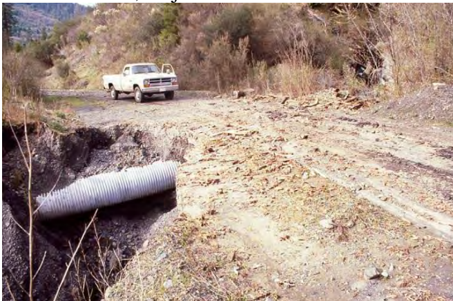
Debris on road; major embankment erosion
