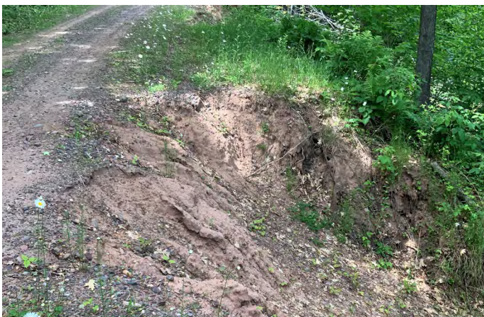
Slumping of the fill
