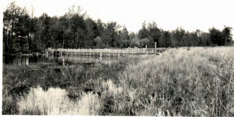
Looking downstream on the Muskegon River weir from a point several hundred feet upstream. Note the flooded, grassy marsh in the foreground (north bank).
