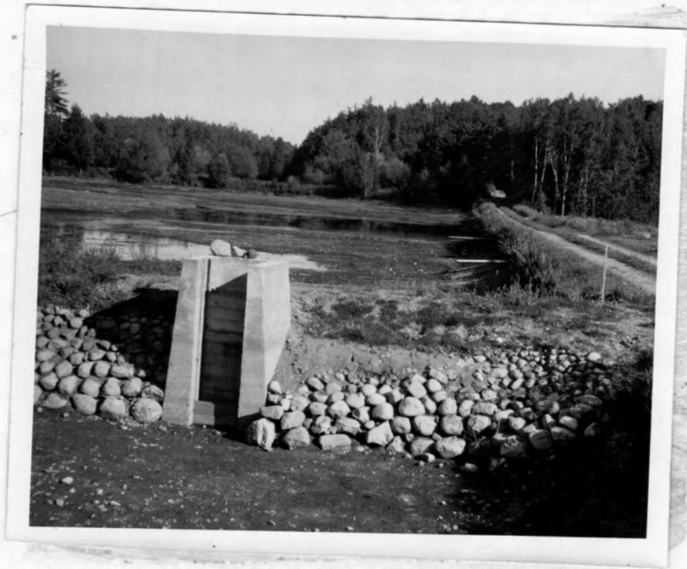
Figure 1. Drained 3 1/2 acre pond at Woodruff Hatchery, Wisconsin, with the outlet structure and seining basin in foreground. Note the hard bottom of the pond and the usual feature of ponds, incomplete draining.
